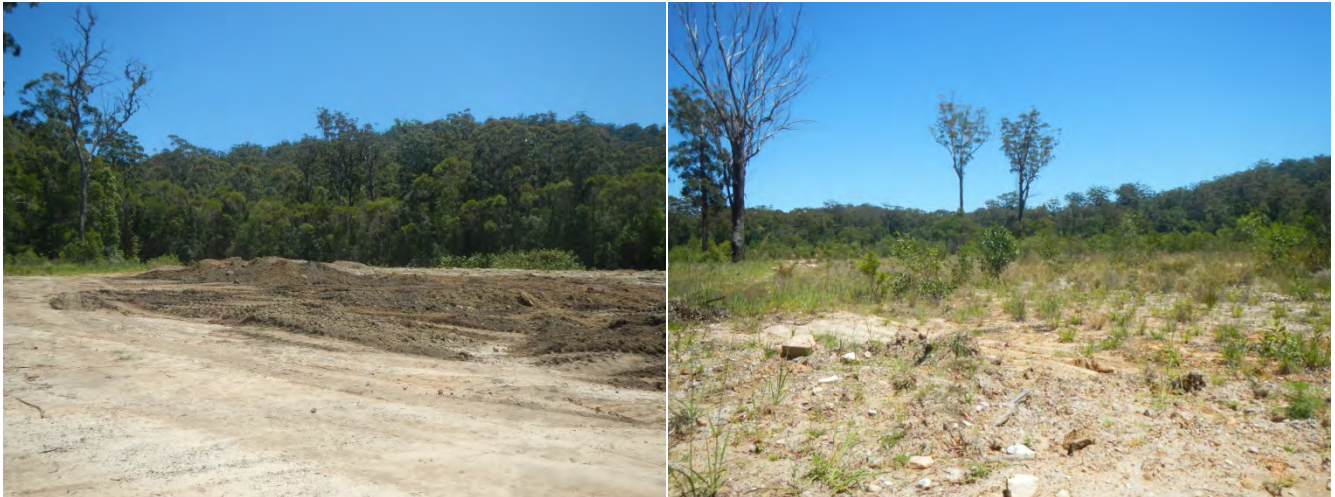
Figures 13 and 14 (left to right): Fill material being spread over past sand mining site and previously rehabilitated land in Site C (refer Figure 1 for location)
