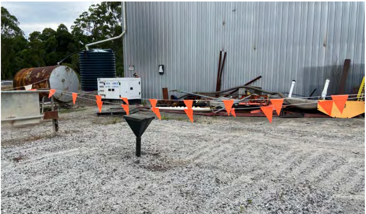
Location of waste oil storage in below-ground 5,000 litre tank - showing pipe/spout for pouring in oil
