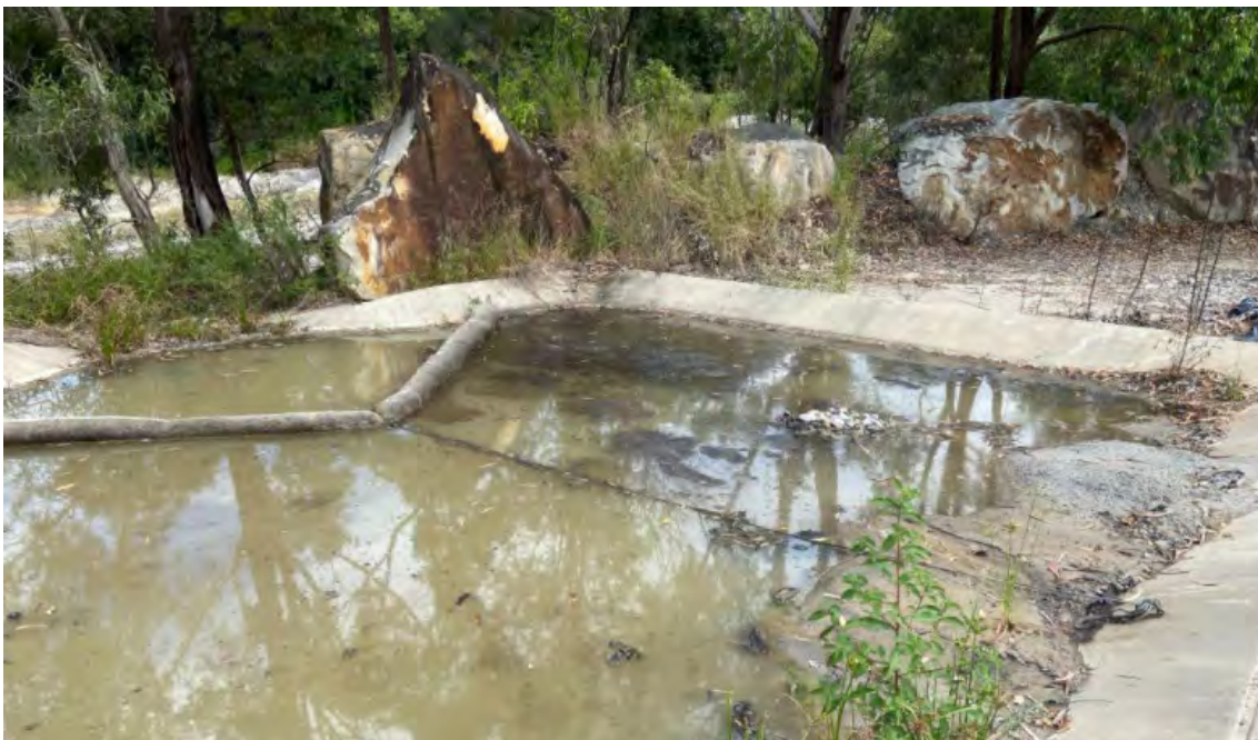
Truck washdown sediment basin
