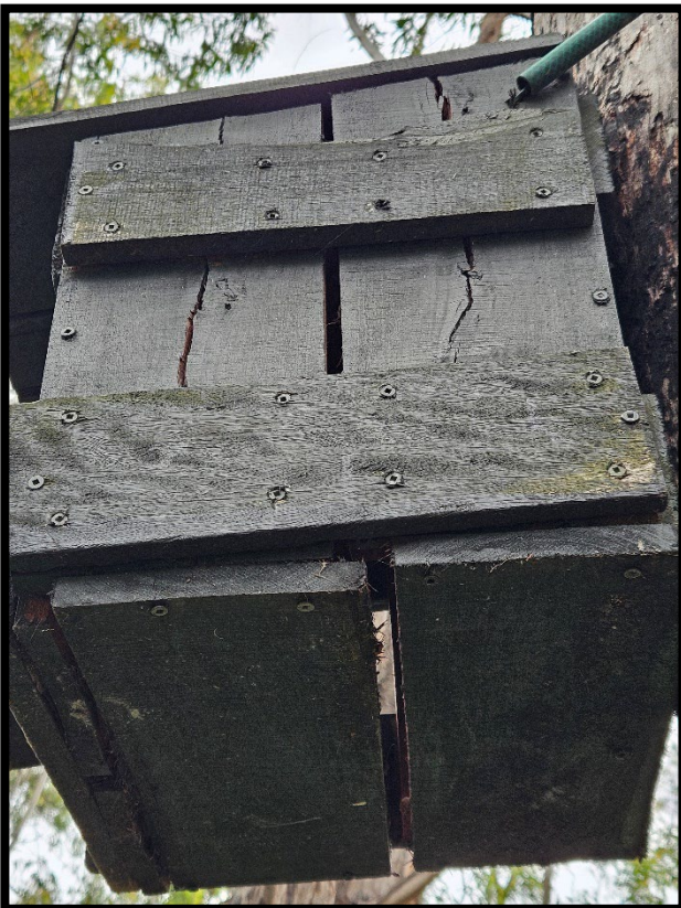
Plate 3-1. Nest box with excessive splits allowing light, rain and wind into the box.
